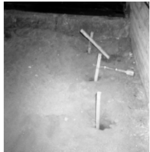
Threaded stud adapter (on ground) will be attached to the screw anchors and lateral anchors. A square plate will be double-nutted onto the adapter and cast in concrete.
