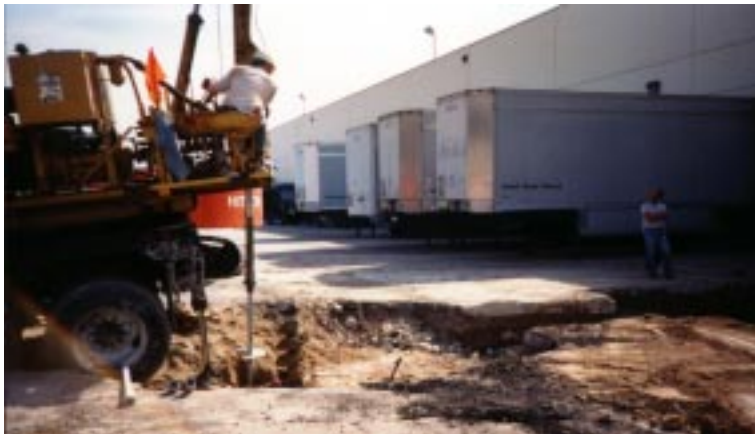
Type SS175 anchors were driven into the ground with a bed mounted digger truck.
